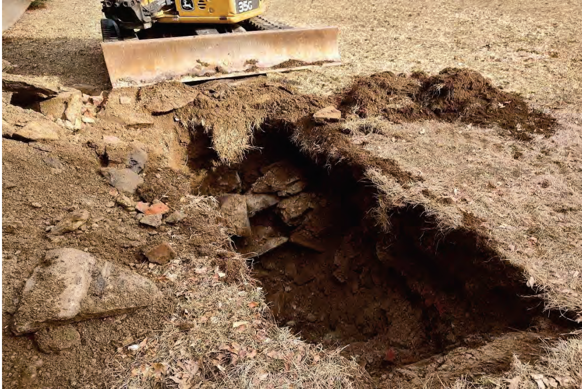
Photo 14: Deep tests, completed by the owner for proposed septic systems show extensive disturbance and building debris to the north of the school building.
