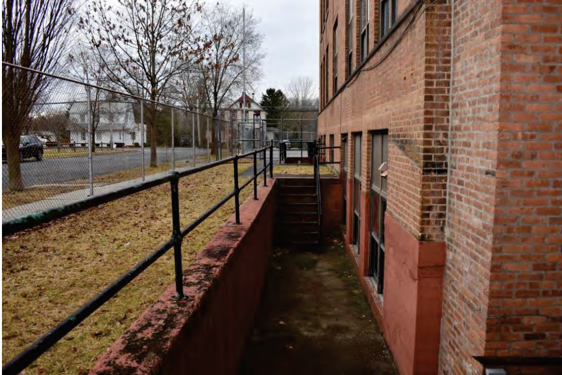
Photo 6: Access points on the eastern side of the building are below grade. View to the south.
